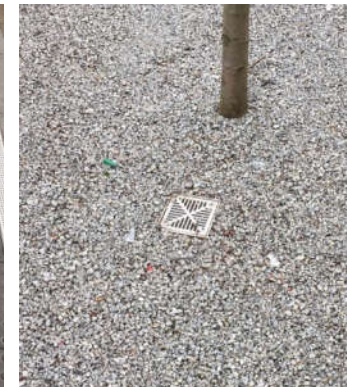
Arboresin or similar to tree pit – where they are location in the footway or carriageway
