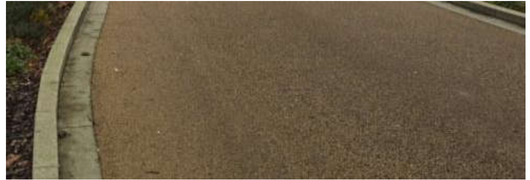
Buff Asphalt or similar – for crossing points, junctions, key points along the street
