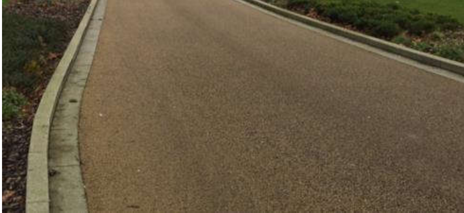
Buff Asphalt or similar – for crossing points, junctions, key points along the street
