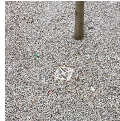
Arboresin or similar to tree pit – where they are location in the footway or carriageway
